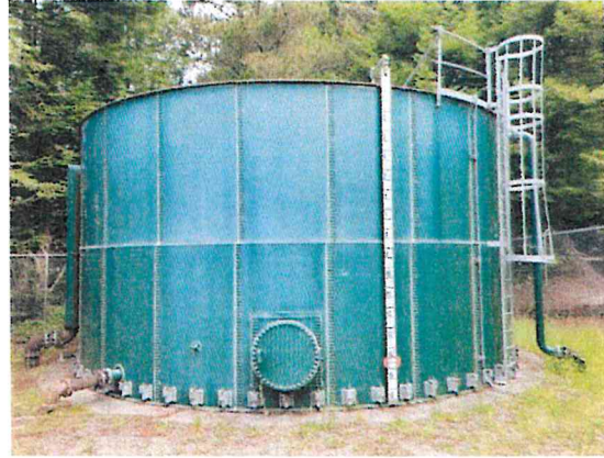
100,000 Gallon Steel Bolted Tank
