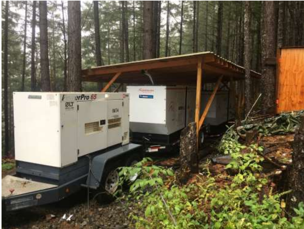
Generators located on scene.
